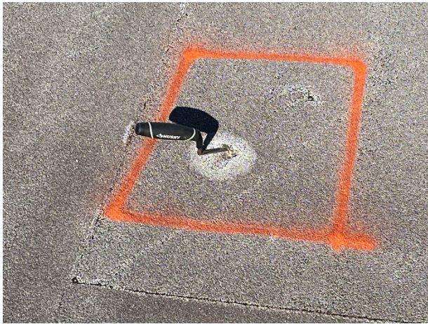
Section B: moisture detected at roof puncture
