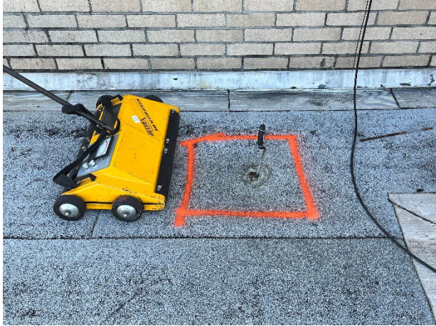
Section B: moisture detected at roof puncture
